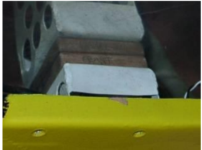
Closeup of Space Occupying Chunk Of Wood (SOCOW)
