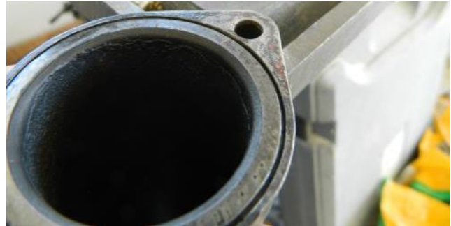
The intake pipe and flange. The surface of the flange and the end of the intake pipe should be in the same plane. They're not—the intake pipe is slightly recessed, maybe about 0.025 inches
